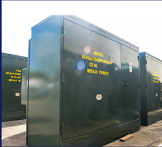
Pad-mounted Distribution Transformers
