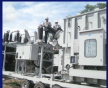
Integrated Compact Substation
